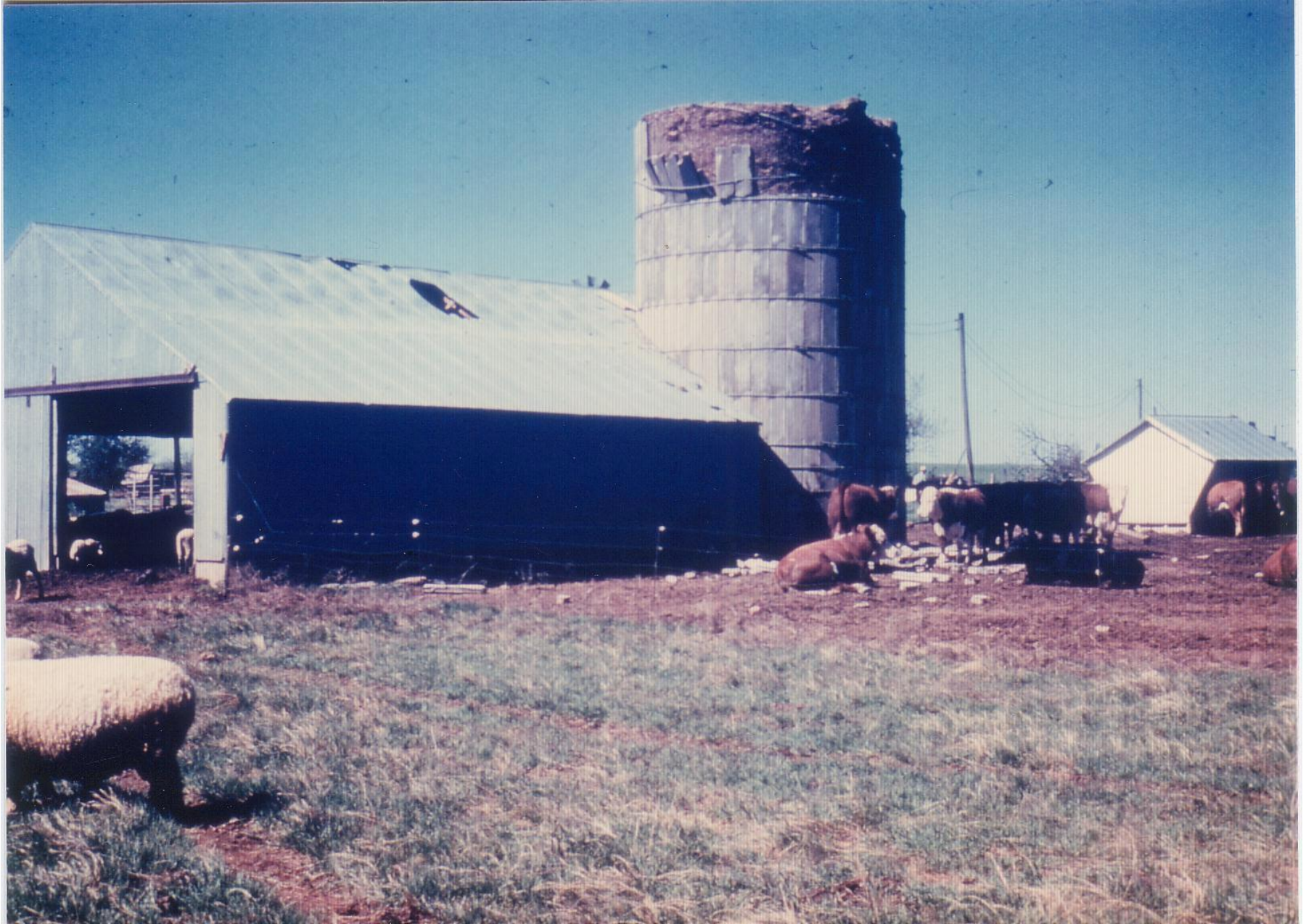
TORNADO0002: Silo shed and silo showing intact ensilage where blocks have been torn away. Feedlot w/clueless steers and self-feeder at far R. None were seriously injured & they stayed inside the electric fence even though no electricity. Sheep @ L & pig shed thru silo shed doors.
