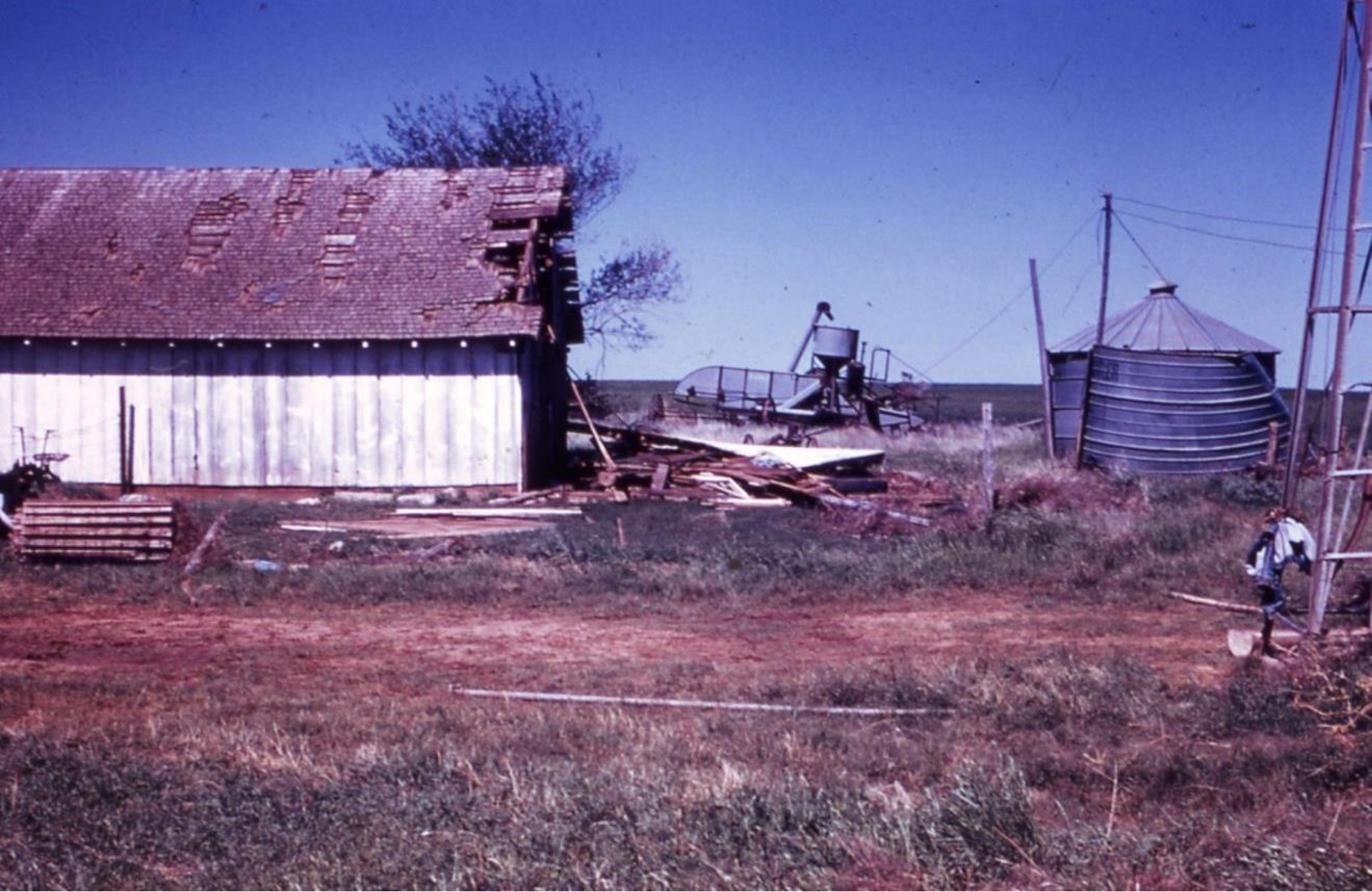
DAT 11-21: Machine shed with missing N side annex, looking W from near pig pen. Note 2 steel grain bins - one distorted w/roof missing, pull-type Case combine, windmill & "water-heater" water trough (far R). Roll of cribbing for top of silo at far L.
