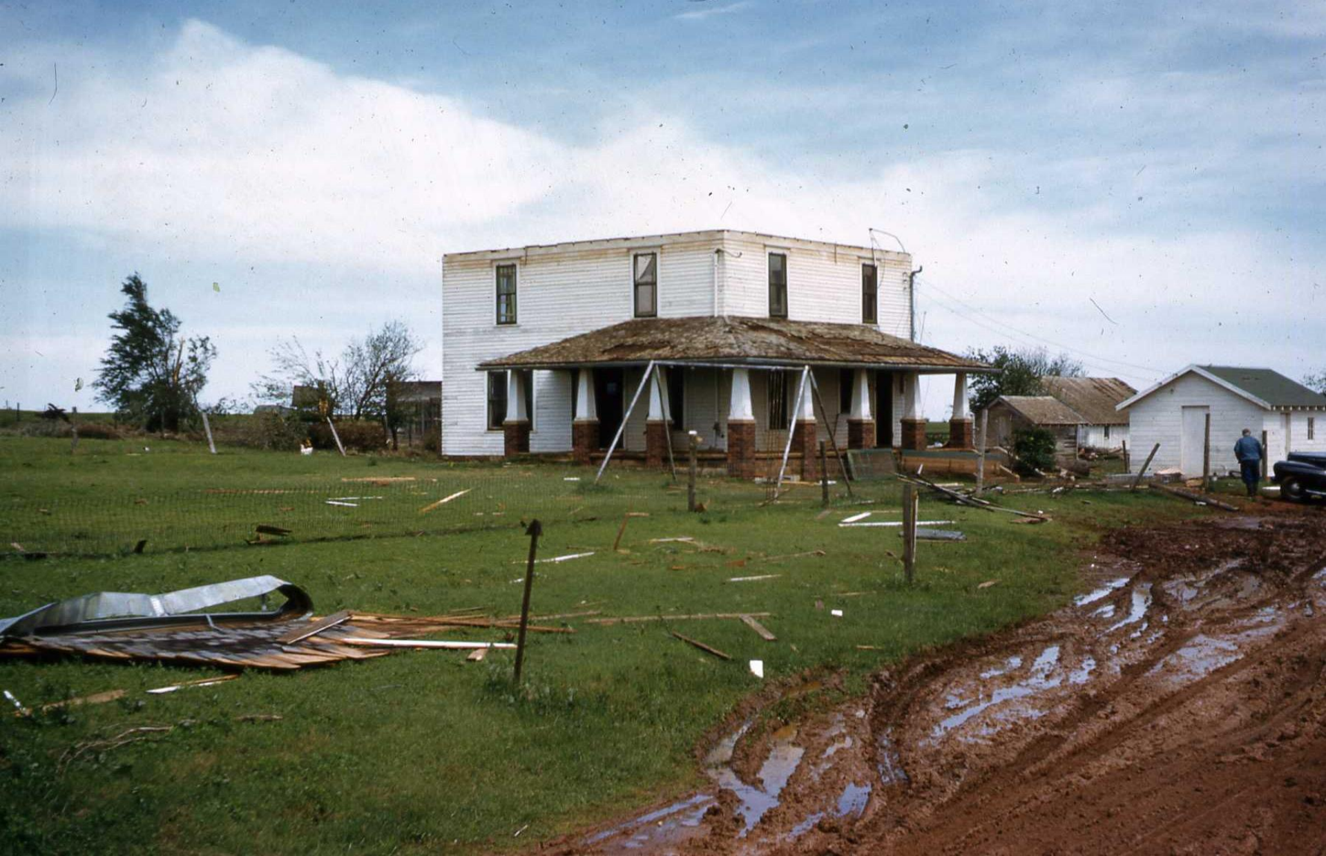
Jake Regier slides: "Tornado damage @ Uncle Dave & Aunt Rosa Toews Farm, April 1962" (sic). Note intact summer kitchen/wash house, mouse house, machine shed, w/ brooder house behind house at L. Chickens too! Piece of house roof w/gutters in L foreground & screen door and porch bench in front.
