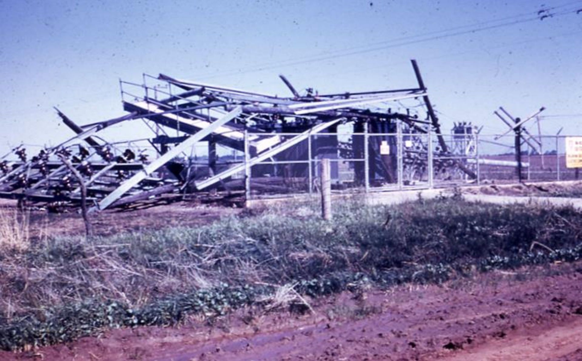
Another view (source unknown) of the destroyed OG&E electric substation @ NE corner of 12 Acres, looking NNW from "Wall Street."
