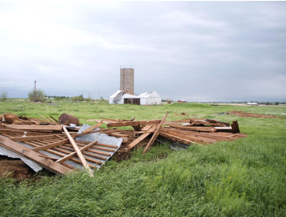
Photos of our destroyed sheep barn after a late summer, 2009 tornado. Our heavily damaged silo shed is at back center in the photo at L.
