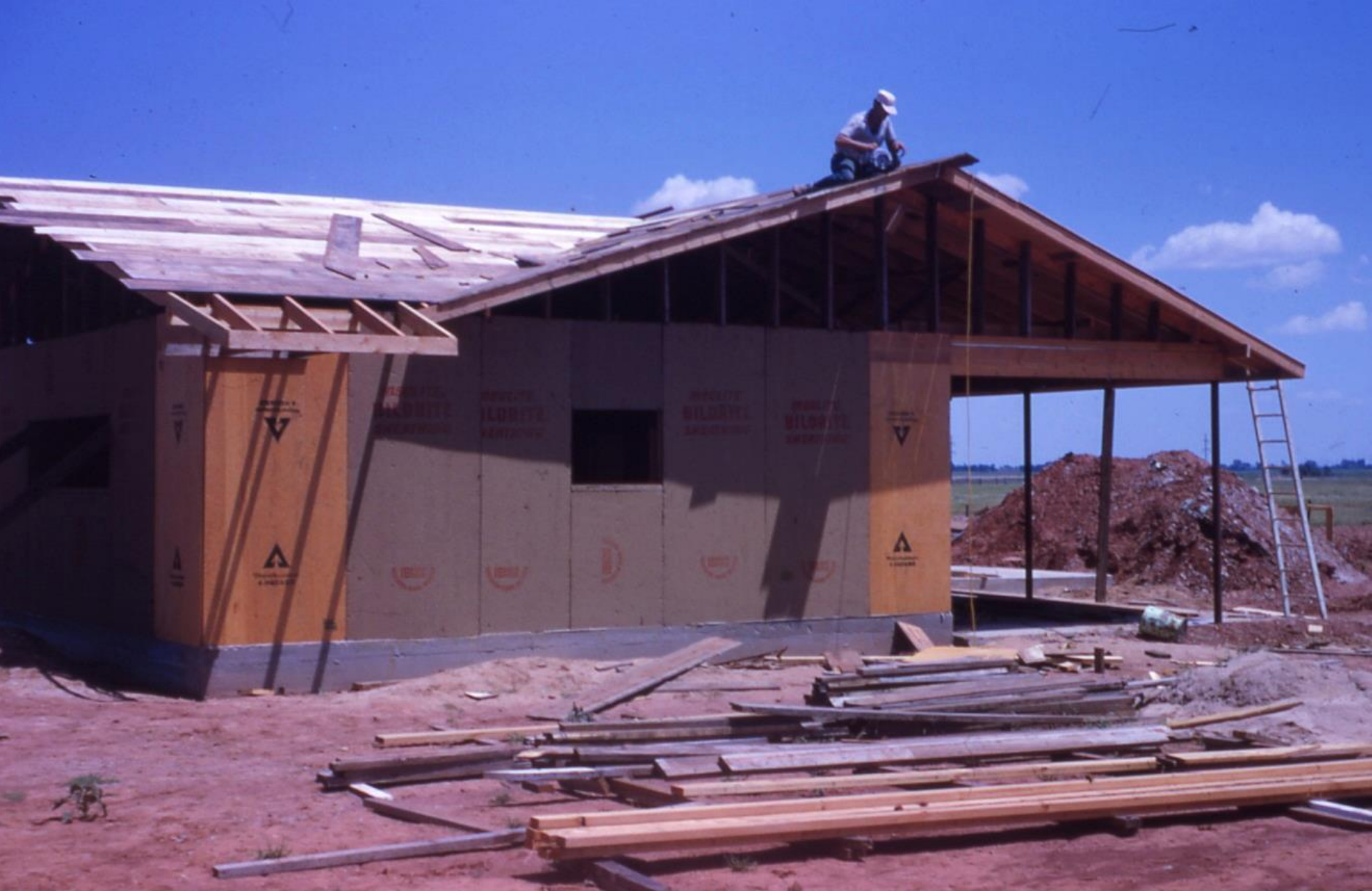
DAT 12-22: We salvaged lots of lumber from the house and barn and pulled lots of nails to build a very nice house along the Kremlin blacktop. Most all of the studs, lots of the floor and ceiling joists, & yes, roof sheathing too (barn siding), were from our house and barn! [~1962-63]
